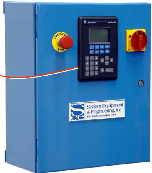
Program-A-Shot control panel
